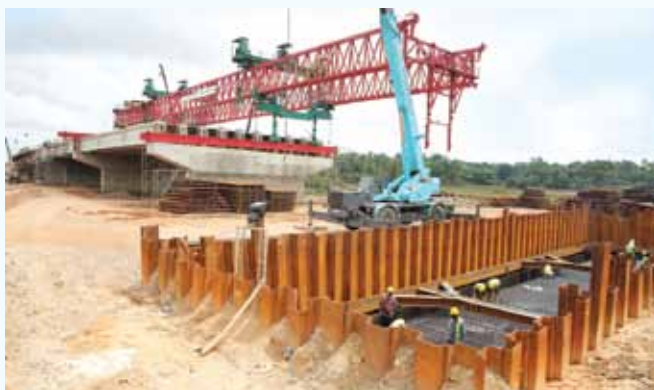
Completion of piling works of the Northern Section of the Colombo Outer Circular Highway
