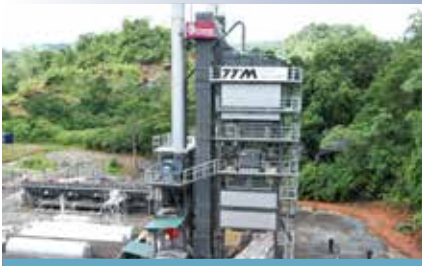
Commissioning of Sri Lanka's largest Asphalt Mixing Plant in Mathugama
