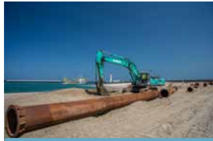
Commencement of construction of the East Container Terminal (ECT) of the Port of Colombo
