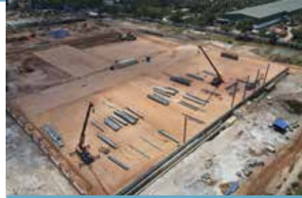
Commencement of construction of the Export Greenfield (EGF) warehousing and logistics facility in Ekala
