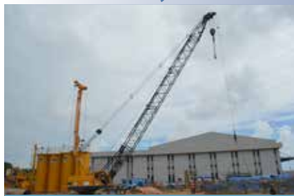
Commencement of construction of the Viaduct for the New Terminal Building at the Bandaranaike International Airport (BIA)
