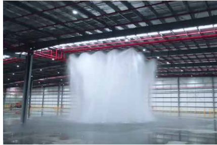
EGF Fire Protection System
